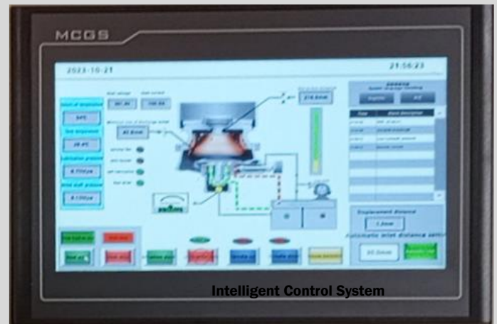
INTELLIGENT CONTROL SYSTEM
